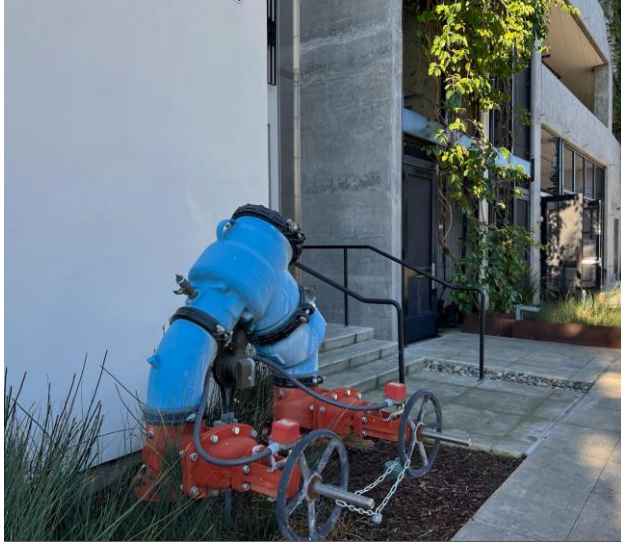
Hidden utilities on the backside of the building (near parking entrance)
