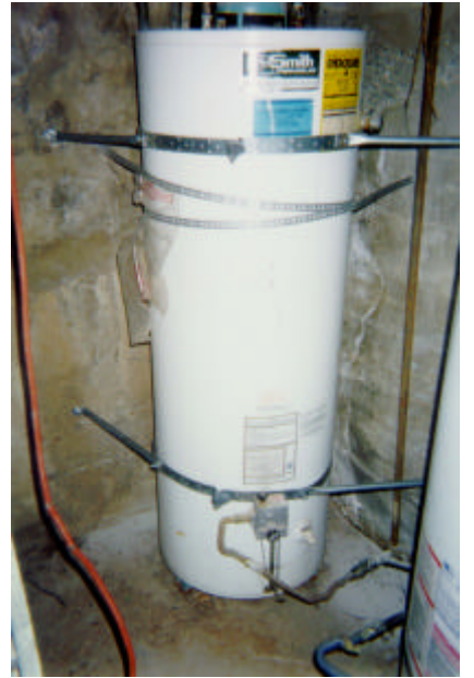
Fig. 7.9 Braced Water Heater
