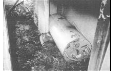
Fig. 7.8 Overturned Water Heater.
