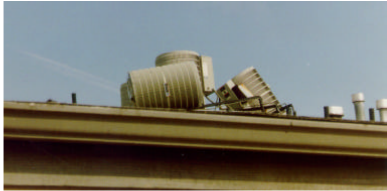
Fig. 7.12 Earthquake Damaged Air Conditioning Units
