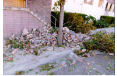
Fig. 7.6 Fallen Brick Veneer
