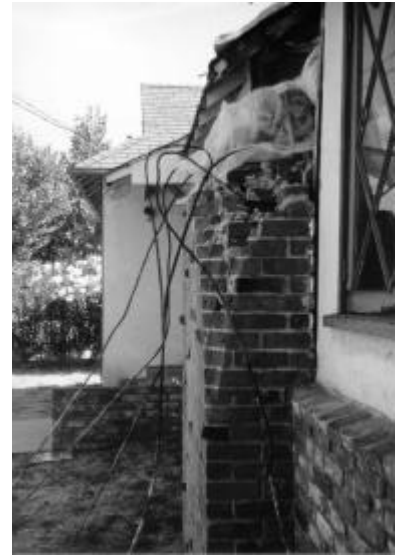
Fig. 7.1 Reinforced Chimney Failure
