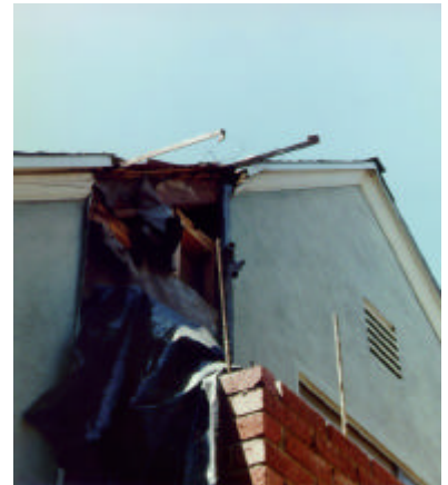
Fig 7.2 Braced Chimney Failure
