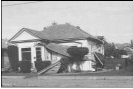
Fig. 7. 4 Porch Roof Collapse.
