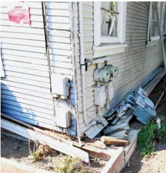
Cripple wall and gas connection failure. South Napa Earthquake. Photo credit: EERI - Petros Keshishian
