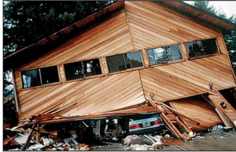
Single Family Home Soft Story Failure, Loma Prieta Earthquake
