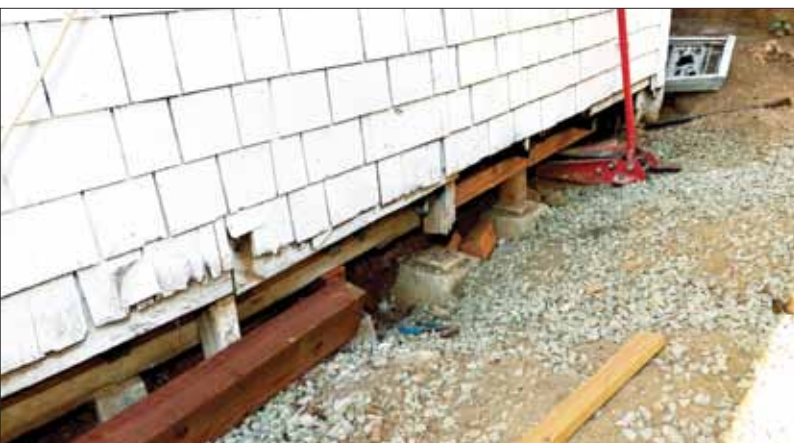
Cripple Wall Failure, South Napa Earthquake
