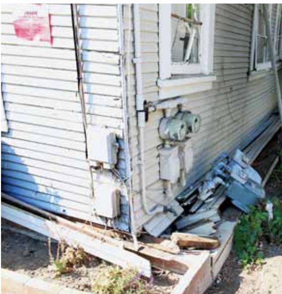
Cripple wall and gas connection failure. South Napa Earthquake. Photo credit: EERI - Petros Keshishian
