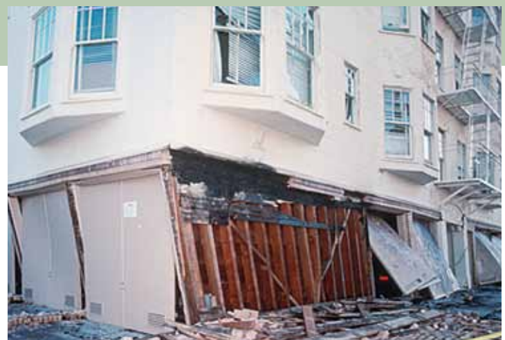
Soft Story Building Failure, Loma Prieta Earthquake
