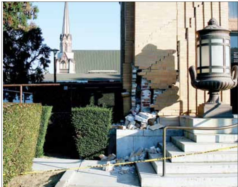
Post Office Building, South Napa Earthquake
