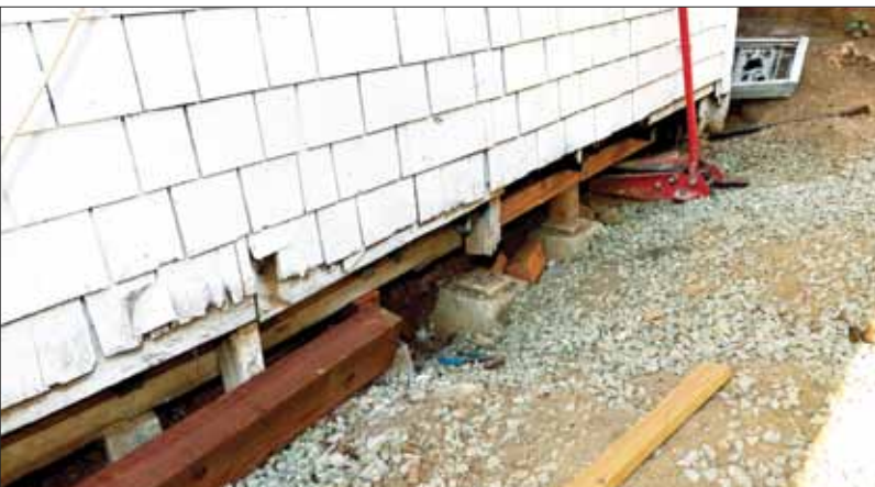
Cripple Wall Failure, South Napa Earthquake
