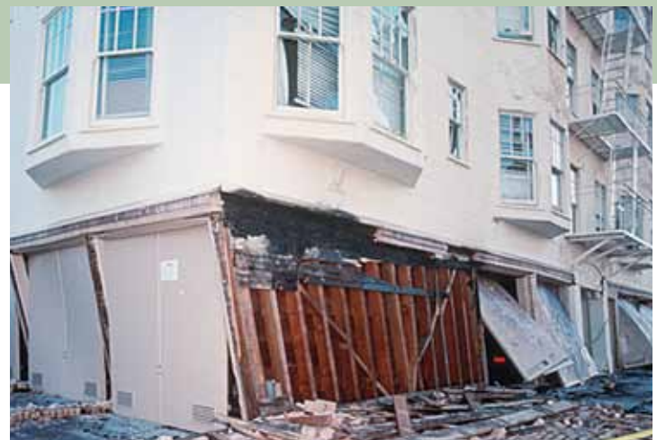
Soft Story Building Failure, Loma Prieta Earthquake
