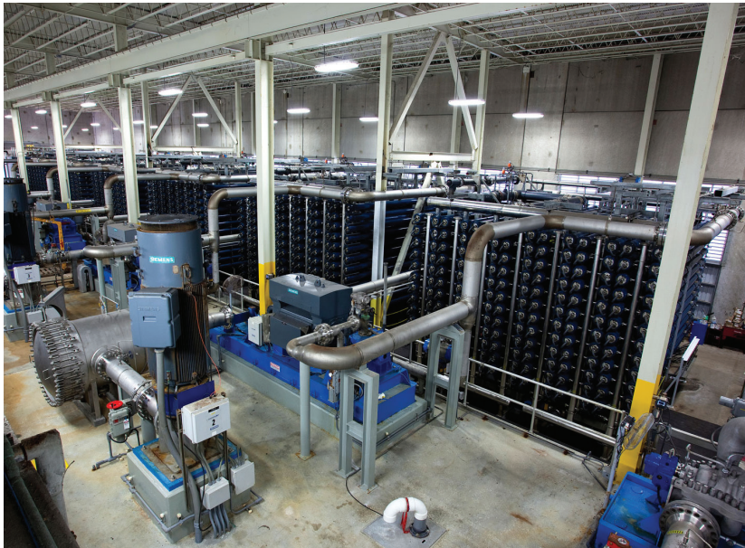
Figure 4.2. The Tampa Bay Seawater Desalination Plant provides up to 25 million gallons of drinking water per day—an important drought-proof, alternative water supply for the region.
