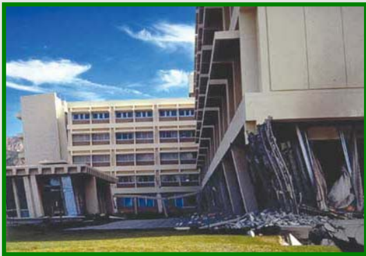
Damage to hospital in 1971 San Fernando Earthquake
