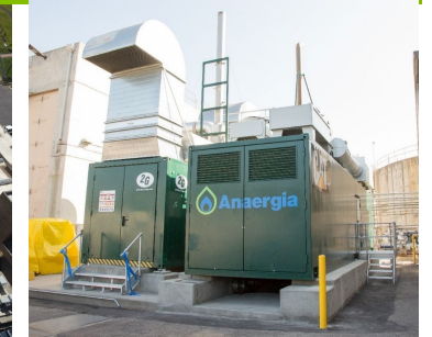
HALE AVENUE RESOURCE RECOVERY FACILITY ESCONDIDO, CA DBOOF
